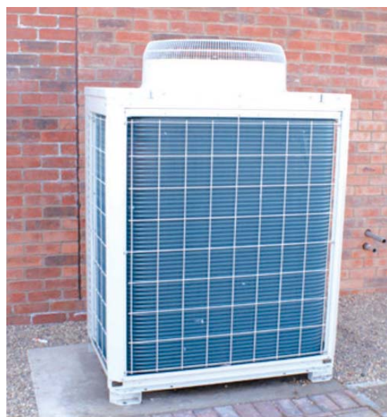
Belaria air source pump, fan and induction unit
